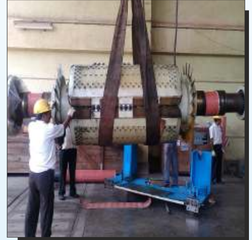
35MVA, Alternator Rotor Threading Out
