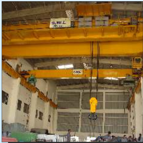
65T, EOT Crane
