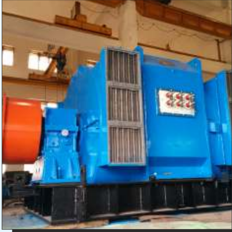
7.5MVA,6.6 KV, Alternator Post Overhauling
