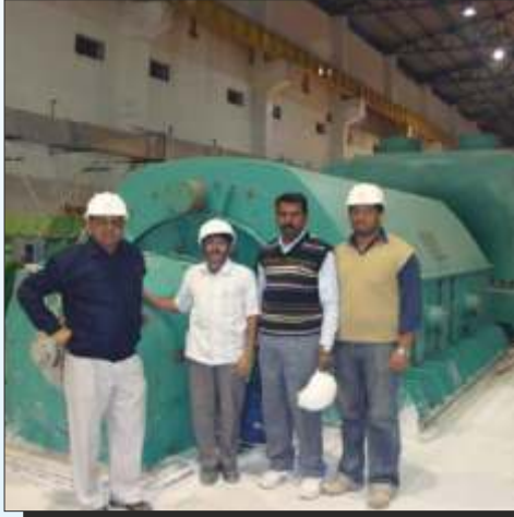
61MVA, Alternator Post Overhauling
