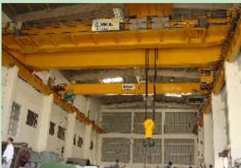
65 TON OVERHEAD CRANE
